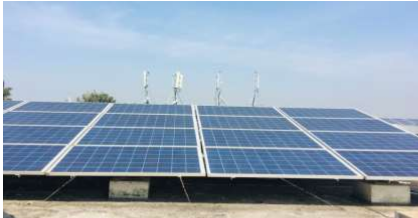
Fig. 1: Rooftop Solar PV Plant Installed at BVRIT
