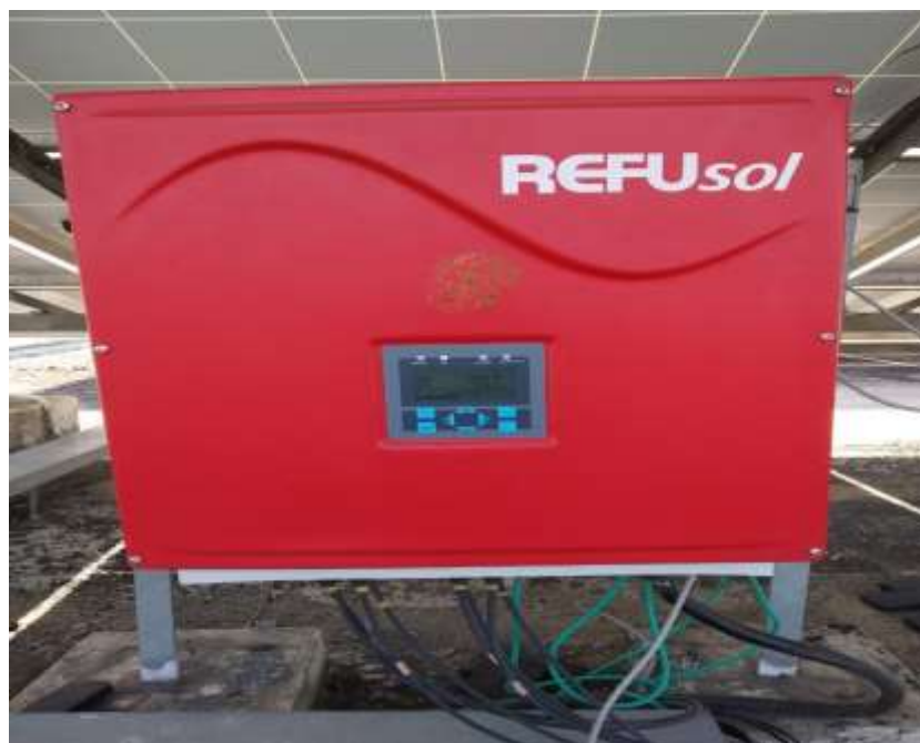
Fig. 2: REFUsol Inverter of 20kW p Capacity
