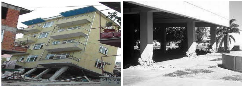
Figure 1: Soft Storey failures
